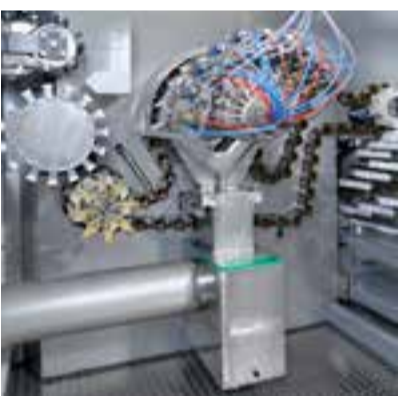
Exhaust performance was optimized through scientific support: Overspray is extracted and fed directly out of the machine room.
