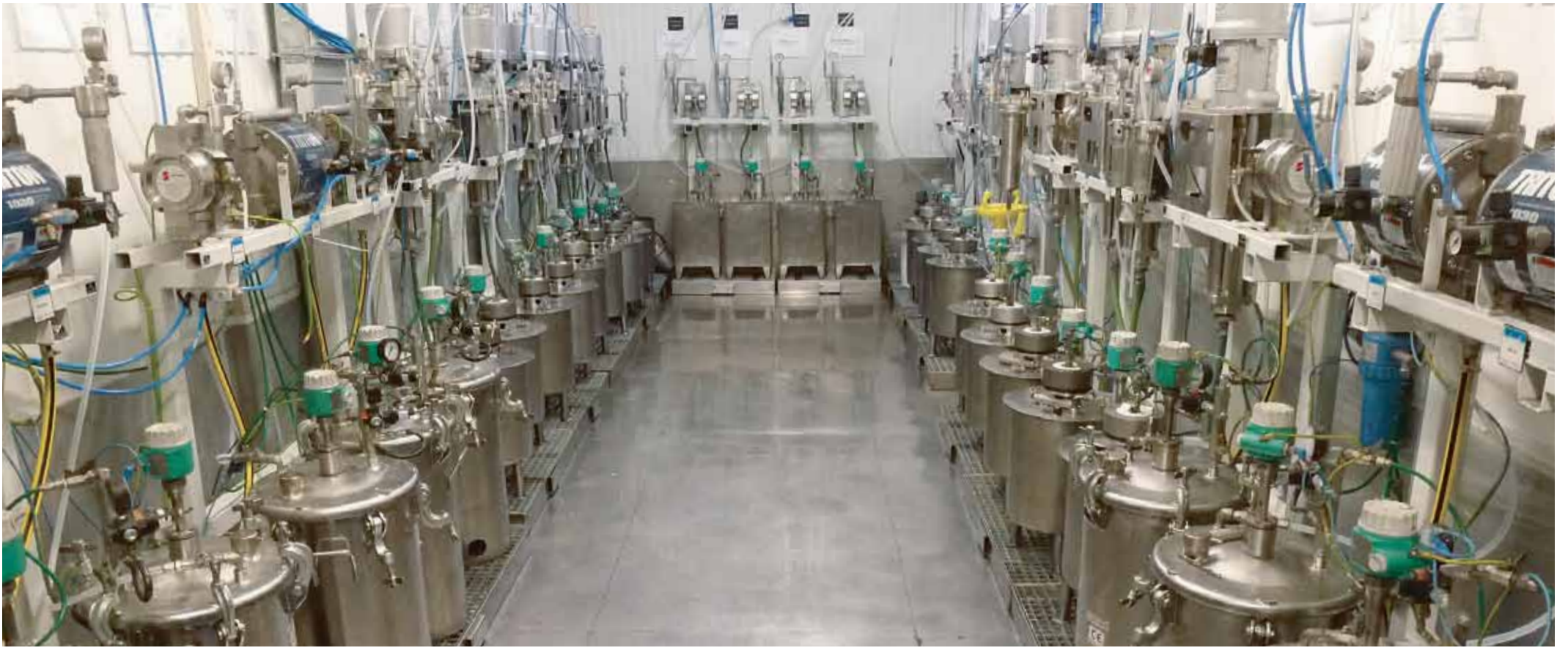
The 43 supply tanks are centrally coordinated and controlled by one software.
